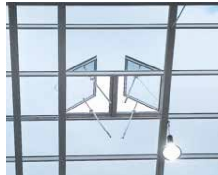
Synchronous control of several drives
