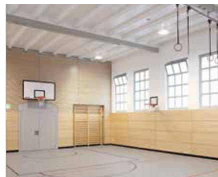
Daily ventilation and smoke exhaust as and when required via chain drives
