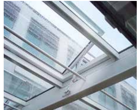
Opening and closing large and heavy skylights
